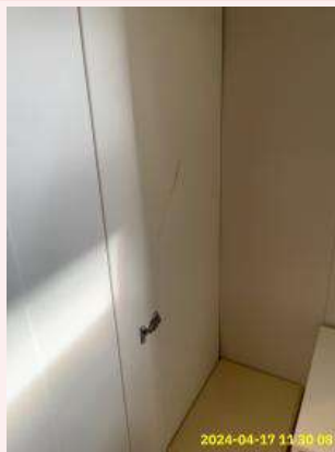
5:12 Furnishings Scratch on the inside wall
