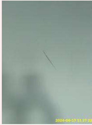
6:1 General Overview Scratches on the entry wall
