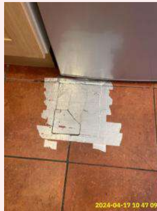
3:1 General Overview Floor damage
