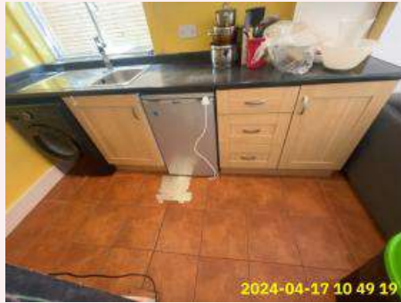
3:3 Flooring Floor damage
