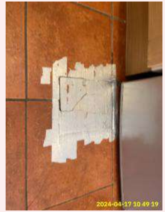
3:3 Flooring Floor damage
