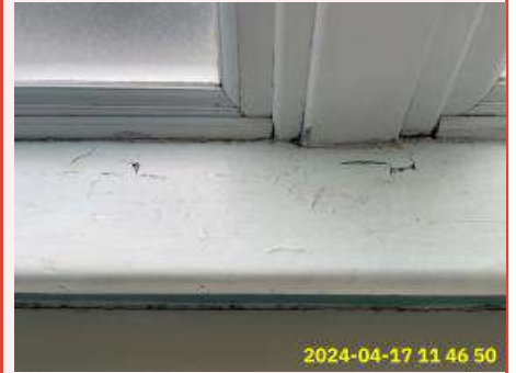
6:9 Windows/ Curtains Scratches on the bottom
