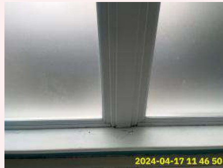
6:9 Windows/ Curtains Scratches on the bottom
