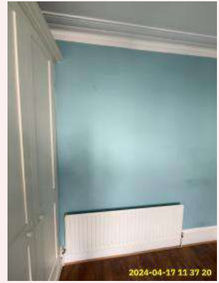
6:1 General Overview Scratches on the entry wall
