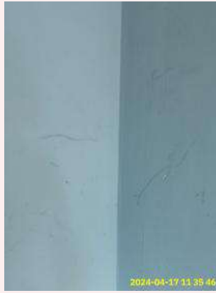
6:1 General Overview Scratches on the entry wall
