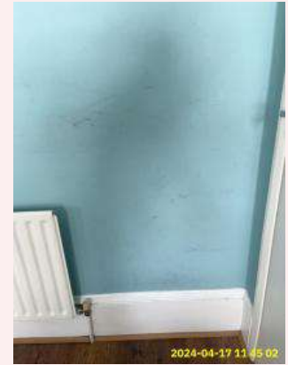
6:8 Walls Scratches on the wall
