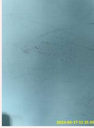
6:1 General Overview Scratches on the entry wall
