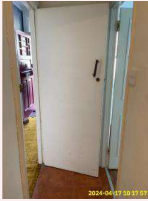
1:3 Doors Scratches on the front door
