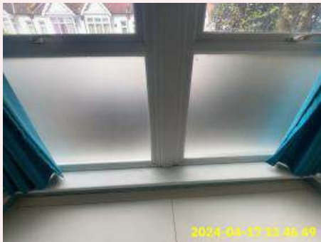
6:9 Windows/ Curtains Scratches on the bottom
