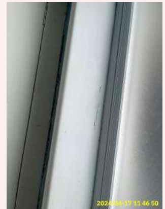
6:9 Windows/ Curtains Scratches on the bottom
