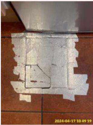
3:3 Flooring Floor damage
