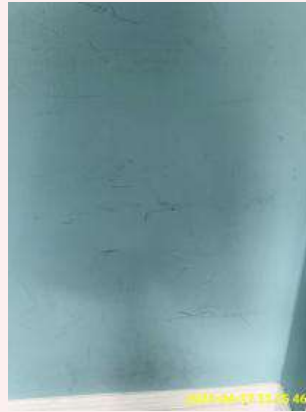
6:1 General Overview Scratches on the entry wall
