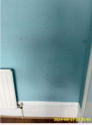
6:1 General Overview Scratches on the entry wall
