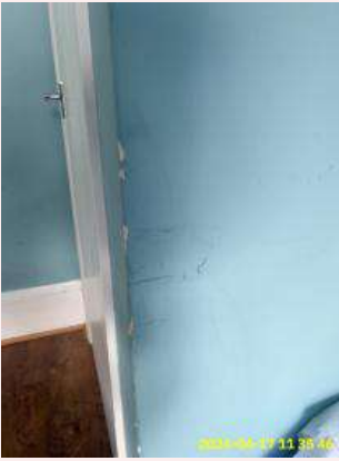
6:1 General Overview Scratches on the entry wall
