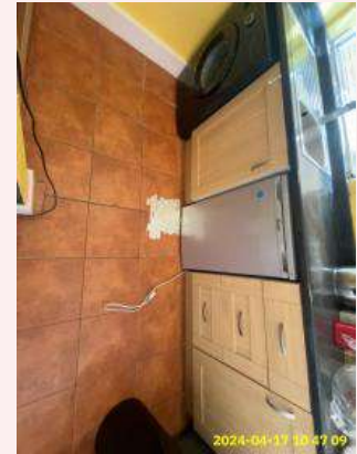
3:1 General Overview Floor damage
