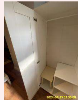
5:12 Furnishings Scratch on the inside wall
