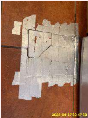
3:1 General Overview Floor damage
