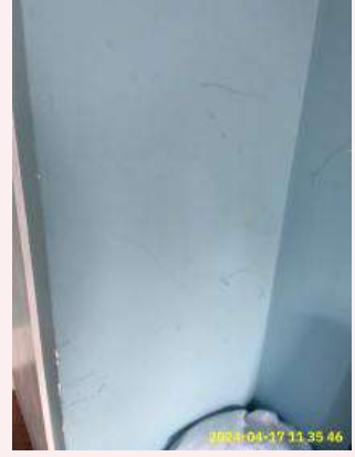
6:1 General Overview Scratches on the entry wall
