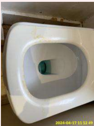
4:9 Toilet Toilet seat stains
