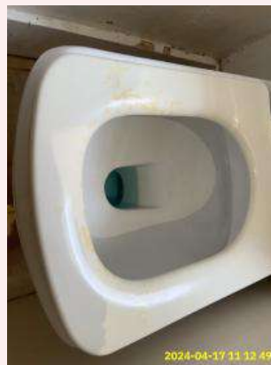
4:9 Toilet Toilet seat stains
