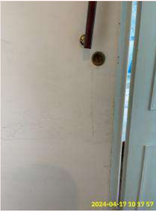
1:3 Doors Scratches on the front door
