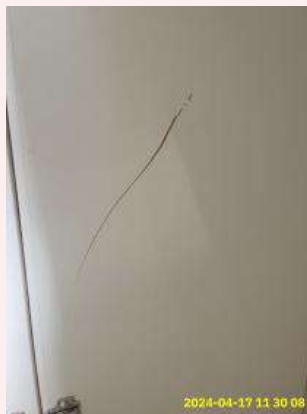
5:12 Furnishings Scratch on the inside wall
