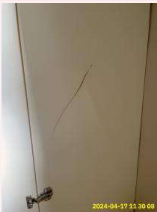
5:12 Furnishings Scratch on the inside wall
