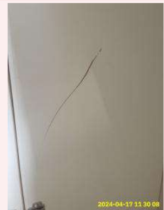
5:12 Furnishings Scratch on the inside wall
