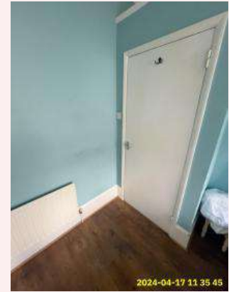
6:1 General Overview Scratches on the entry wall
