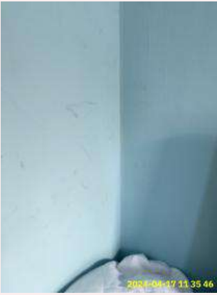
6:1 General Overview Scratches on the entry wall
