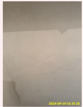
2:14 Storage Seems Dampness; Crack
