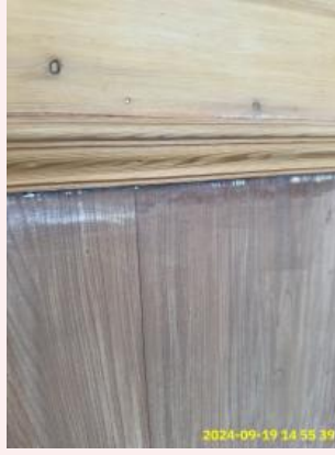
5:3 Doors Paint Marks- Wear and Tear
