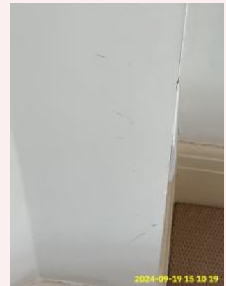
6:8 Walls Crack & Scuff Marks- Wear and Tear
