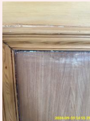
5:3 Doors Paint Marks- Wear and Tear
