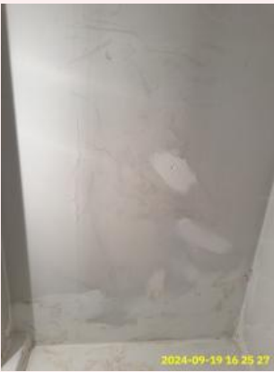
2:14 Storage Seems Dampness; Crack
