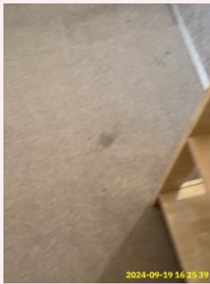
2:14 Storage Seems Dampness; Crack
