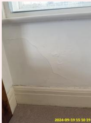
6:8 Walls Crack & Scuff Marks- Wear and Tear
