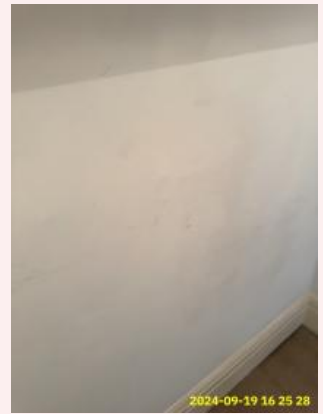
2:14 Storage Seems Dampness; Crack
