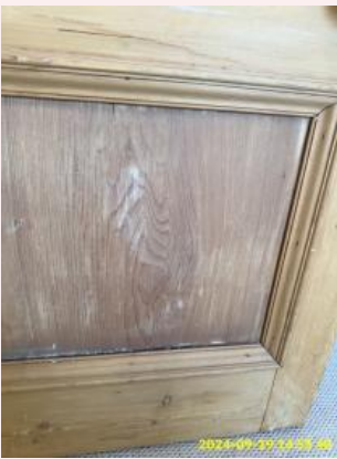
5:3 Doors Paint Marks- Wear and Tear
