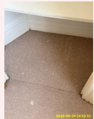
5:11 Storage Room Stain
