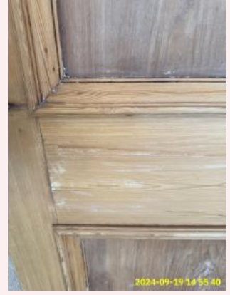
5:3 Doors Paint Marks- Wear and Tear
