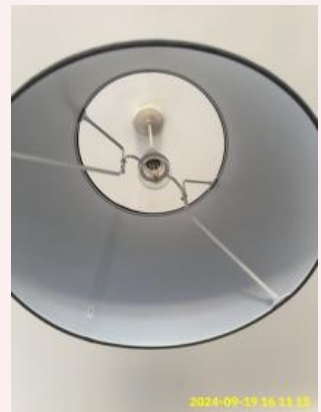
2:6 Lighting Not Working - Tenant Maintenance
