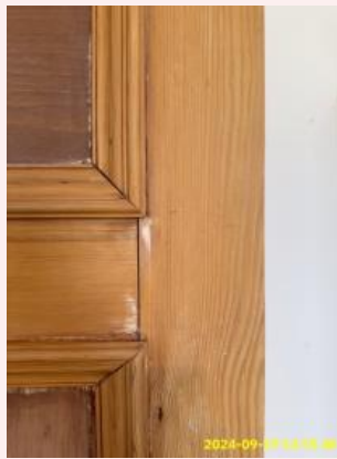
5:3 Doors Paint Marks- Wear and Tear
