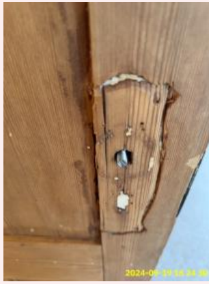
2:14 Storage Damage/KNob Missing - Tenant Maintenance
