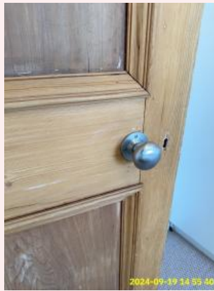
5:3 Doors Paint Marks- Wear and Tear
