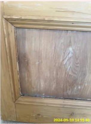
5:3 Doors Paint Marks- Wear and Tear
