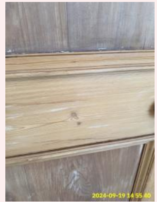
5:3 Doors Paint Marks- Wear and Tear
