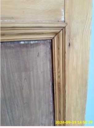
5:3 Doors Paint Marks- Wear and Tear
