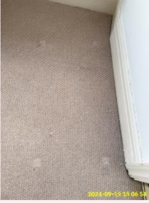
6:4 Flooring Stain - Tenant cleaning
