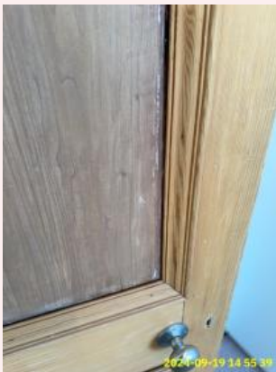
5:3 Doors Paint Marks- Wear and Tear
