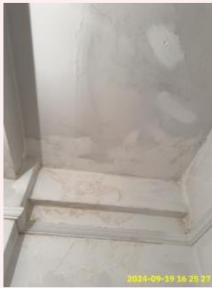
2:14 Storage Seems Dampness; Crack
