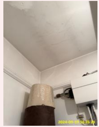
2:14 Storage Seems Dampness; Crack
