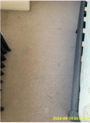
6:4 Flooring Stain - Tenant cleaning
