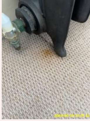
6:4 Flooring Stain - Tenant cleaning
