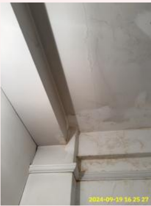
2:14 Storage Seems Dampness; Crack
